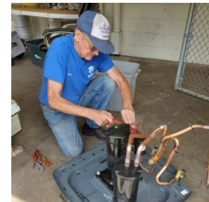
Frank, a dedicated volunteer, stripping an HVAC unit to retrieve the recyclable metals
